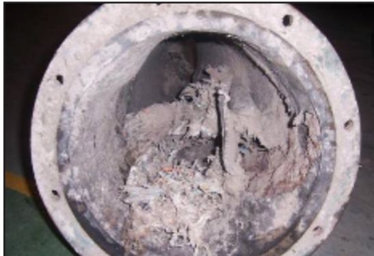
Rubber liner at 3 months
